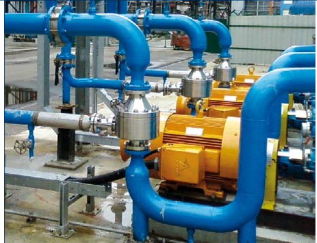
SureFlo ARC valves in a boiler feedwater application
